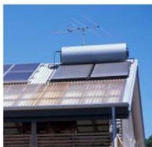
SOLAR WATER HEATER
